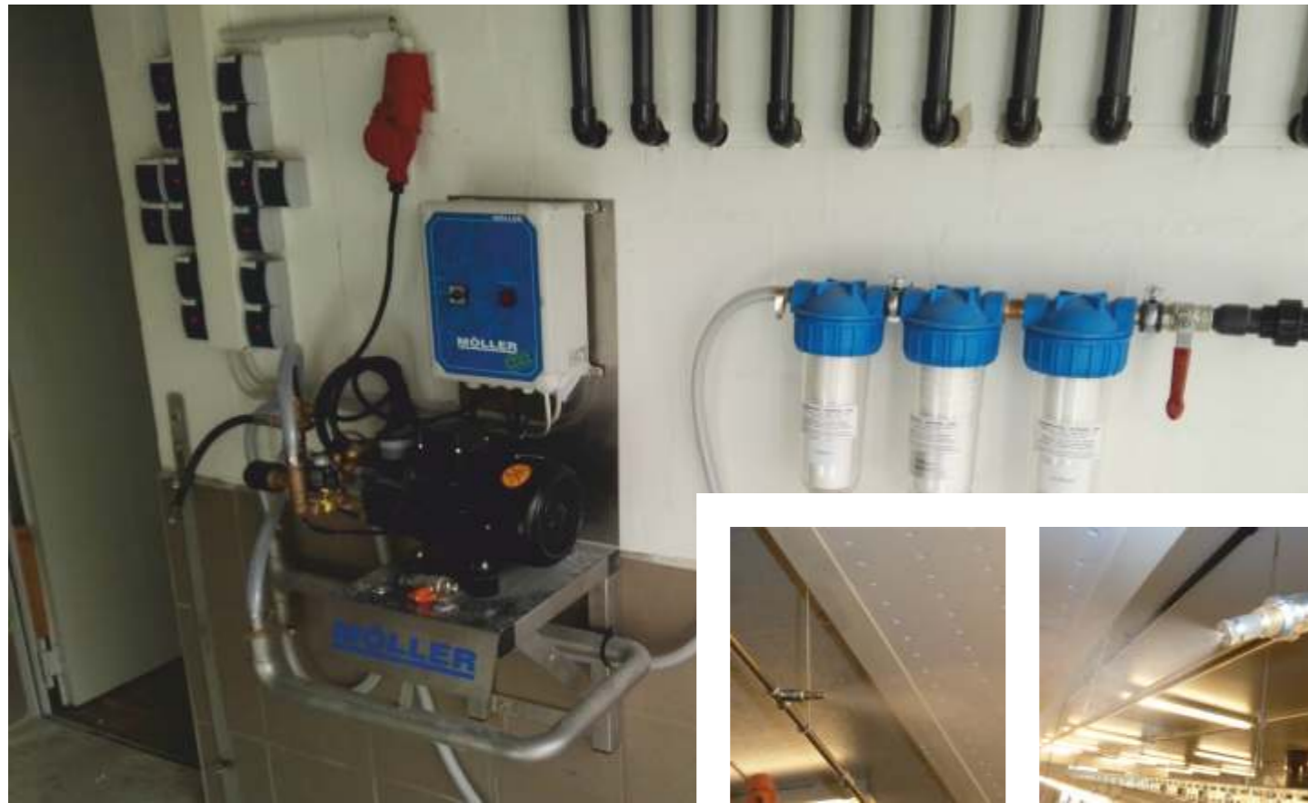
High pressure cooling system
