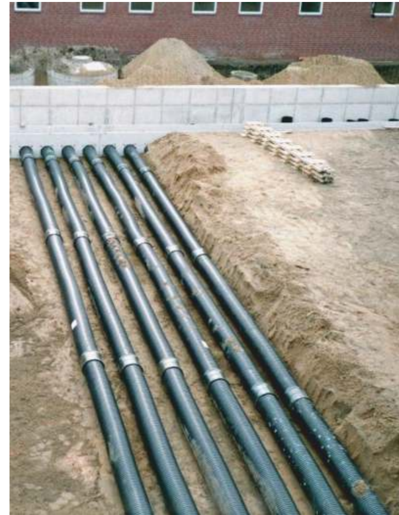
Geothermal pipe system
