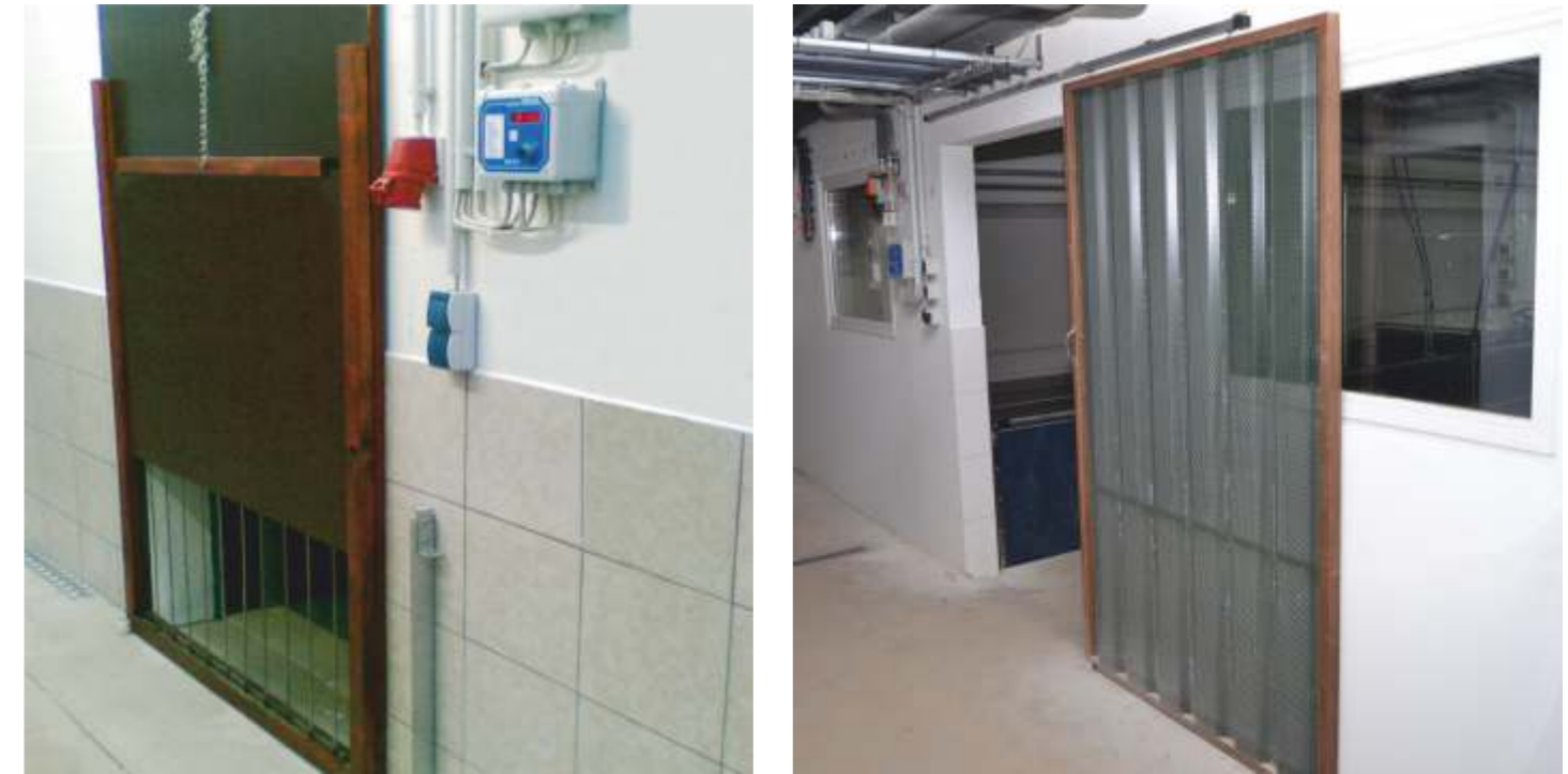
Corridor ventilation system
