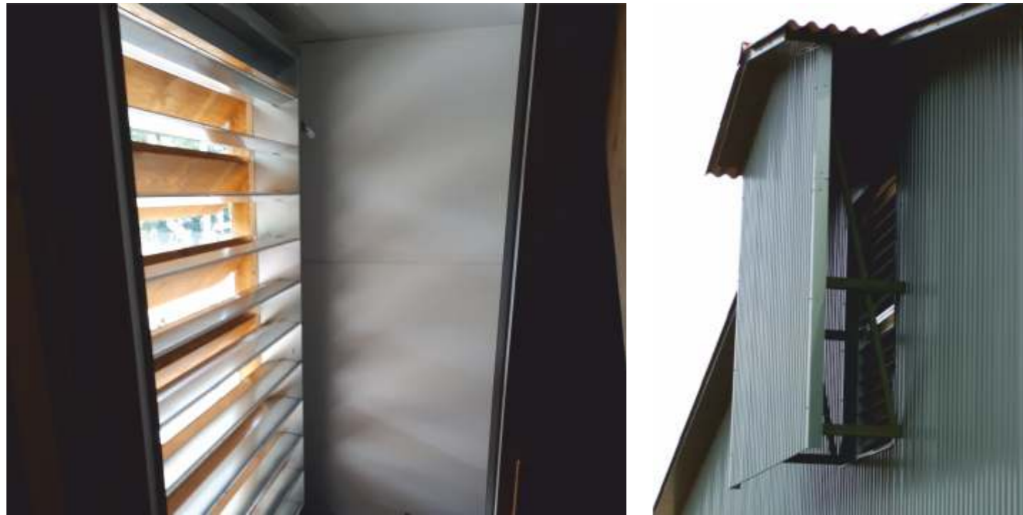
Fresh air supply entry
